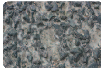
A35: Before preservation
