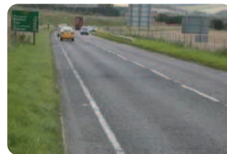
A35: Before preservation
